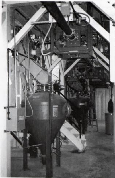
A dense-phase conveyor's pneumatic transfer vessels can either load mixers with ingredients or transport finished batches to packaging.
