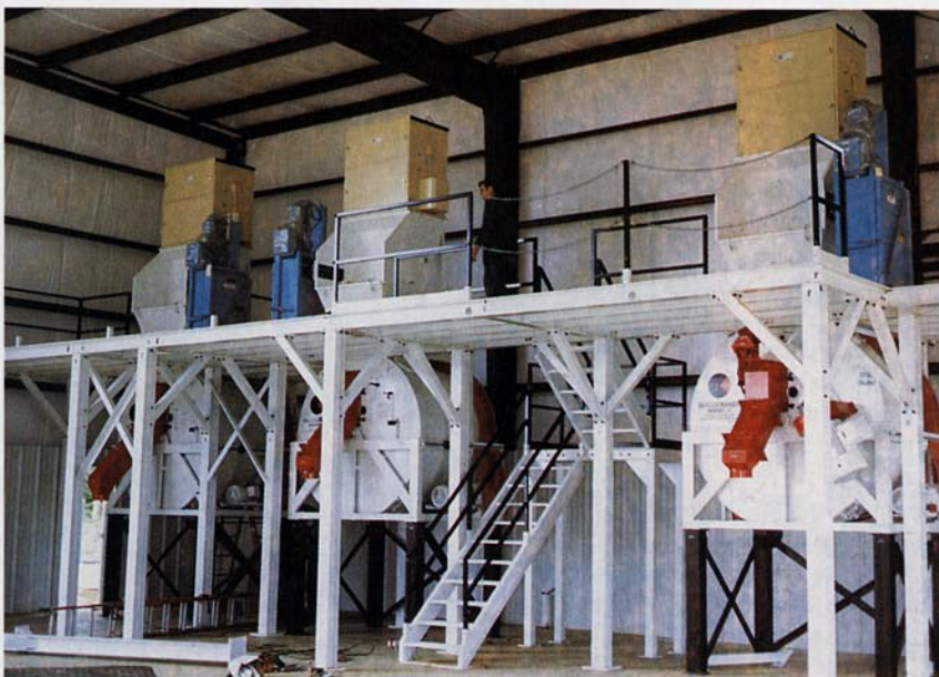
Mixers are supported below bag-dump stations, shown here just after installation and before facility startup.
